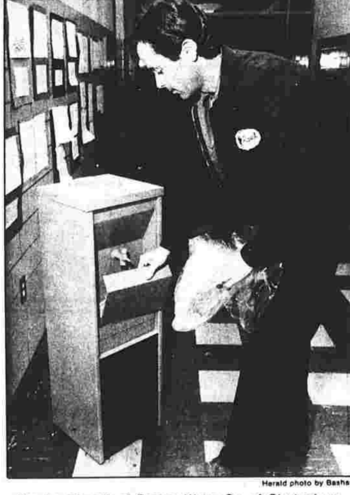
Charles Dimock of Pequot Water Co. of Glastonbury puts a portable bottled water unit in place Wednesday at the Bolton Elementary School.
